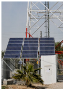
Alcatel Lucent wind and solar technology on a cell site in Qatar
